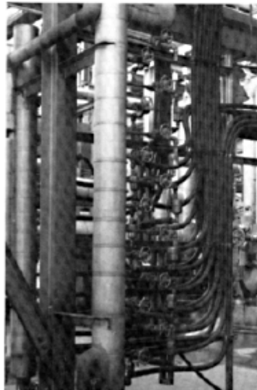
Figure VI Condensate returns to vertical header allow for innovative space savings, too expensive for conventional systems.
