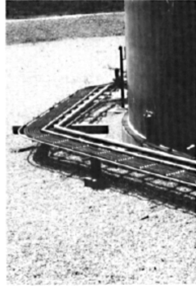
Figure XIII Horizontal ladder type cable tray used for support on long field runs.
